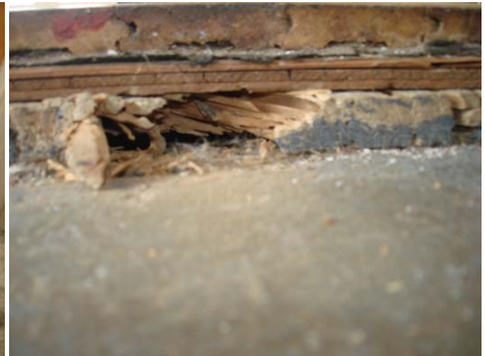
Damage at edge of living room floor.
