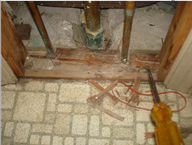
Damage at rear bathroom.
